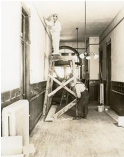
Original Caption: Civil Works Administration, State Project No. 14. Project located in the County of Florence. Project Classification: Public Building Improvement. Photographer: Chris A. Lind. Local ID: 69-CWA-75 (National Archives Identifier: 431966313 ).
