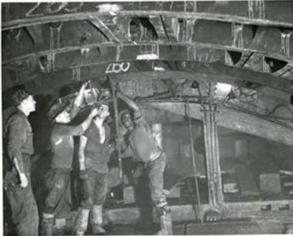
Original Caption: Setting up bolts of a new arch at the tunnel heading during the construction of the Hudson-Midtown Tunnel, New York. Local ID: 69-PWA-1794 (National Archives Identifier: 431966119 ).
