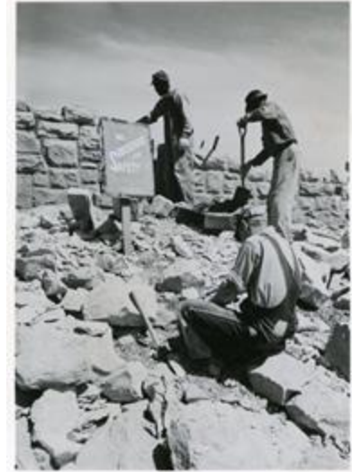
Original Caption: Oklahoma, Perry. Stadium being built entirely by the WPA. Photo shows construction work on the stands and the men wearing safety devices. Local ID: 69-PT-234-23110 (National Archives Identifier: 431966315 ).
