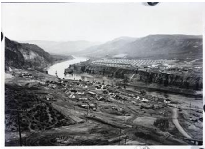
Original Caption: General view of the Grand Coulee Dam site. Local ID: 69-PWA-2023B (National Archives Identifier: 434070818 ).
