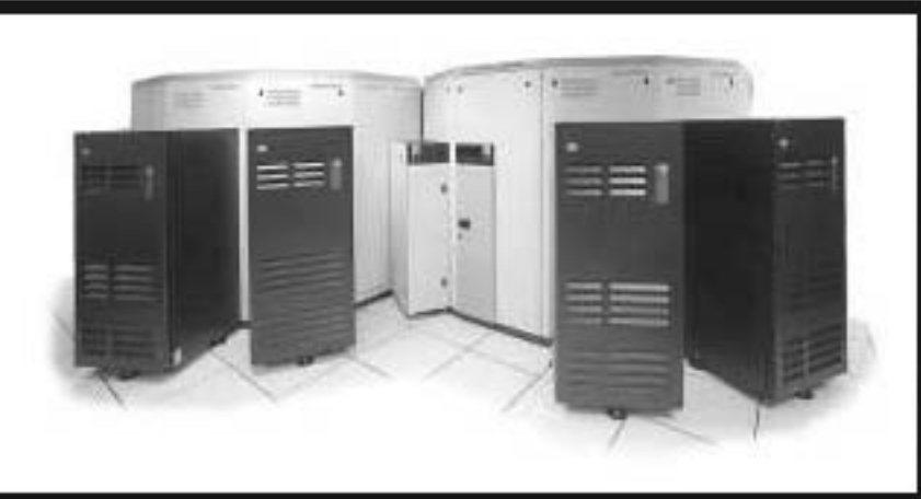
Two of the three StorageTek 9310 tape silos at SDSC. Each silo holds up to 6,000 tapes, and each tape can hold up to 20 GB of data. (Courtesy, SDSC)
