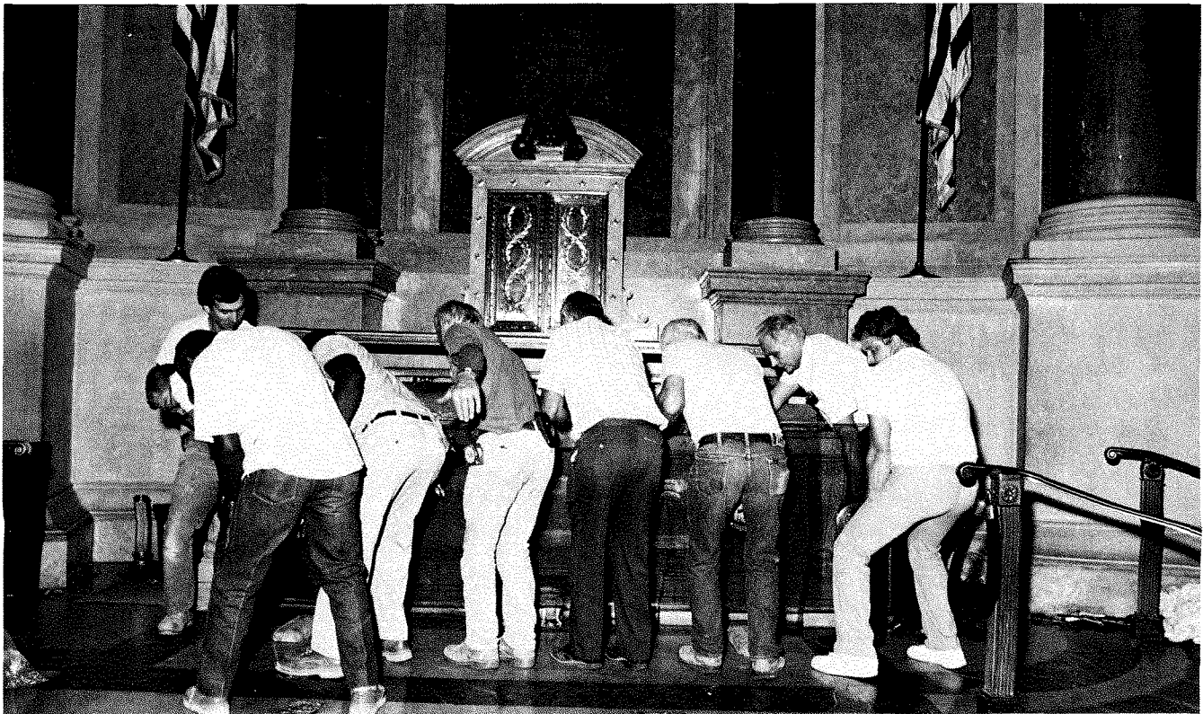
Contractors install a permanent laminated glazing in the bronze exhibition case above the Constitution and Bill of Rights. The ballistics-tested material provides added security for the Charters of Freedom and allows distortion-free viewing of the documents while filtering out potentially damaging ultraviolet radiation. (Photograph by Nancy Olds.)
